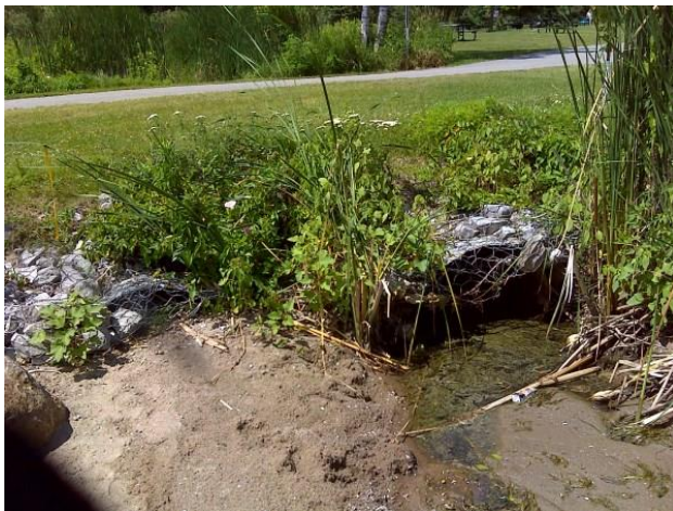
Photo 7: Outlet of Park Road flow at Innisfil Beach/ Lake Simcoe. Two culverts, one with sediments obstructing flow.
