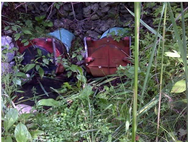
Photo 9 : Outlets from WTP to overflow channel.
